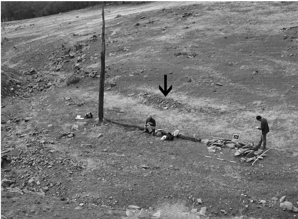
Figure 79. Building platform, Feather River, Butte County. Excavation into the hillside created a level surface. The arrow indicates stone terracing (Photograph by ASC, Sonoma State University).
